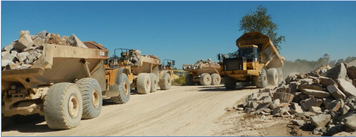
Discharge of bulk rock in the primary jaw crusher.
